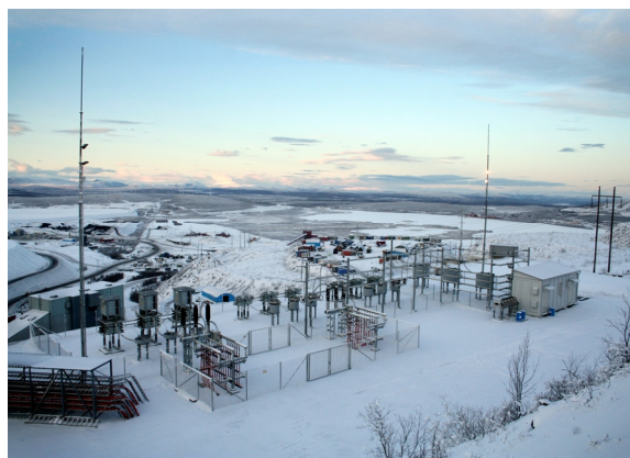
Picture 3. LKAB SVC system
